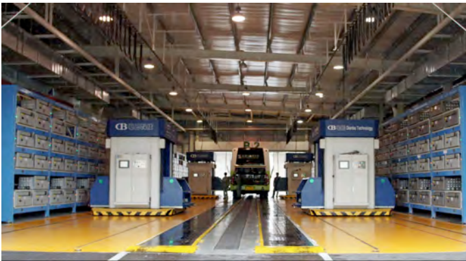
Fig. 6. A Huge-scale Battery Exchange Station. (Without this, battery buses cannot be operated.)
