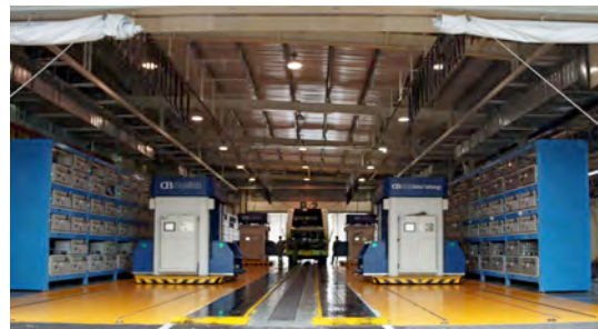
App. Fig. 2. A large-scale battery exchange station. (Without this, battery buses cannot be operated.)
